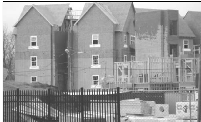
In September, the Borough held the ground breaking ceremony for the student housing portion of the Rowan Blvd. project. This picture shows the progress as of December 2008 with the majority of the exterior construction completed.
